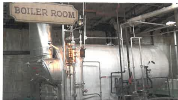
Image 14: Boiler Machine at the Boiler Room (Resource No. 23)
