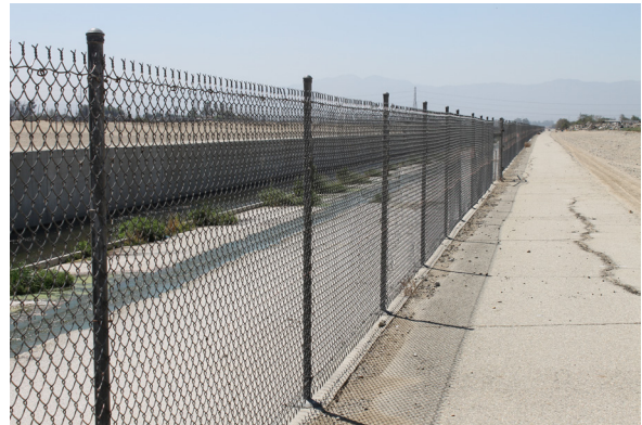
Cucamonga Creek Flood Control Channel and Flood Control Basin located east of the project site.
