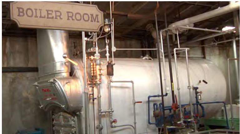
Image 14: Boiler Machine at the Boiler Room (Resource No. 23)
