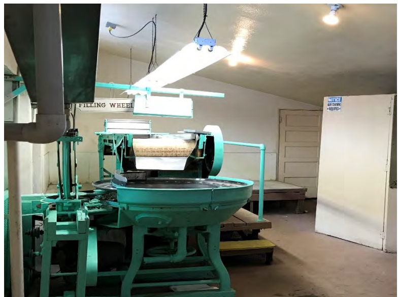
Image 8: Filling Room showcasing the Filling Machine (Resource No. 21).
