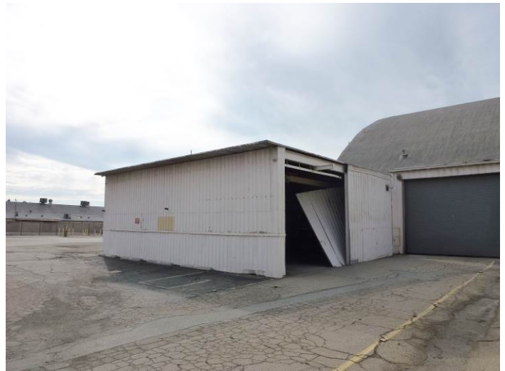
Image 12. View looking south at the northwest and northeast façades of the Wash Building.
