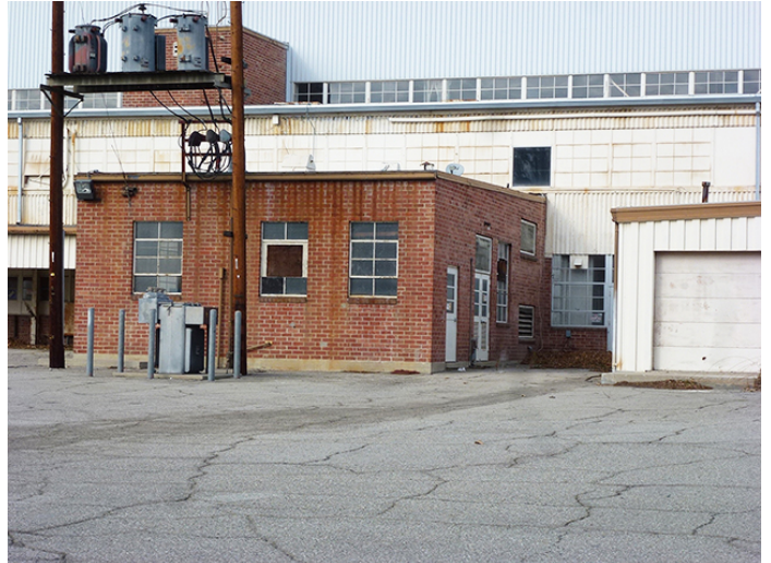
Image 6. View looking northwest at the south and east facades of the Diesel Tanks room.
