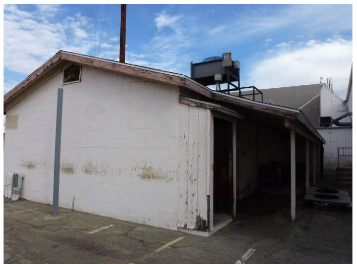
Image 8. View looking north at the southwest and southeast façades of Building J.
