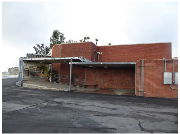
Image 20. View looking northwest at the south façade of the USO building (formerly the West Lobby).
