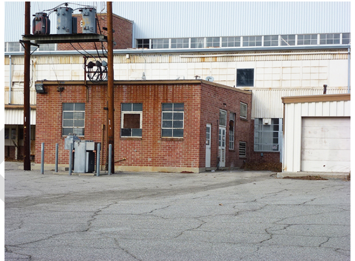
Image 6. View looking northwest at the south and east façades of the Diesel Tanks room.
