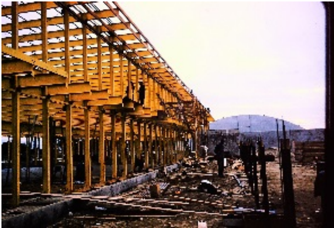
Image 9. View looking northeast at the south façade, ca. 1956. Source: Collection of Colin Russell.
