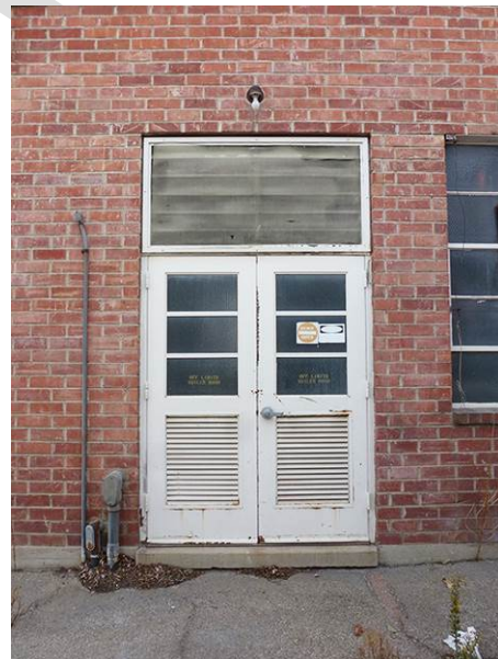
Image 8. Detail view of the entrance on the east façade of the Diesel Tanks room.
