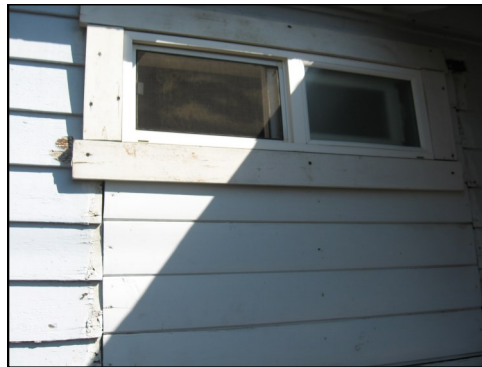
Example of an inappropriate bathroom alteration
