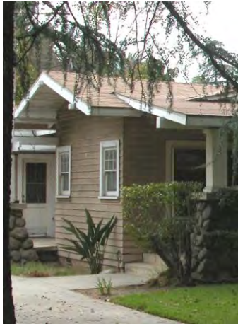
Low slope roof with large, exaggerated overhangs with wood supports and fascia.
