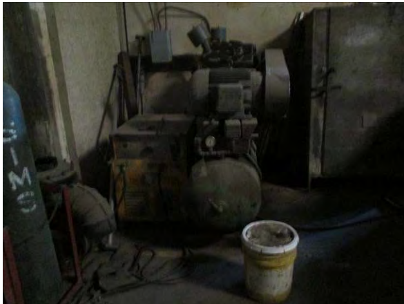
Photo #13 View of the air compressor located in the warehouse.
