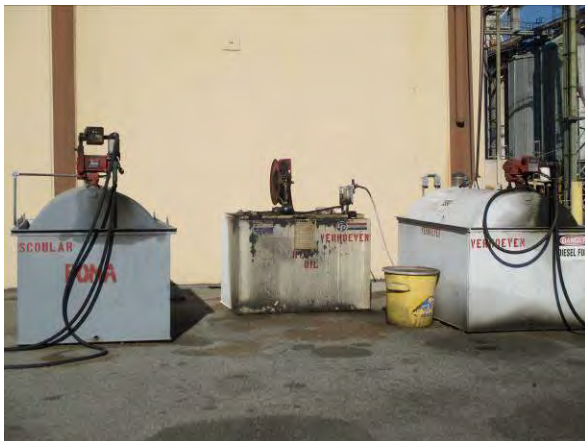
Photo #15 View of three ASTs located on the exterior eastern side of the office/warehouse building.
