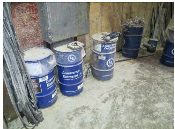
Photo #24 View of the 30-gallon drums of lubricant located in the mill.
