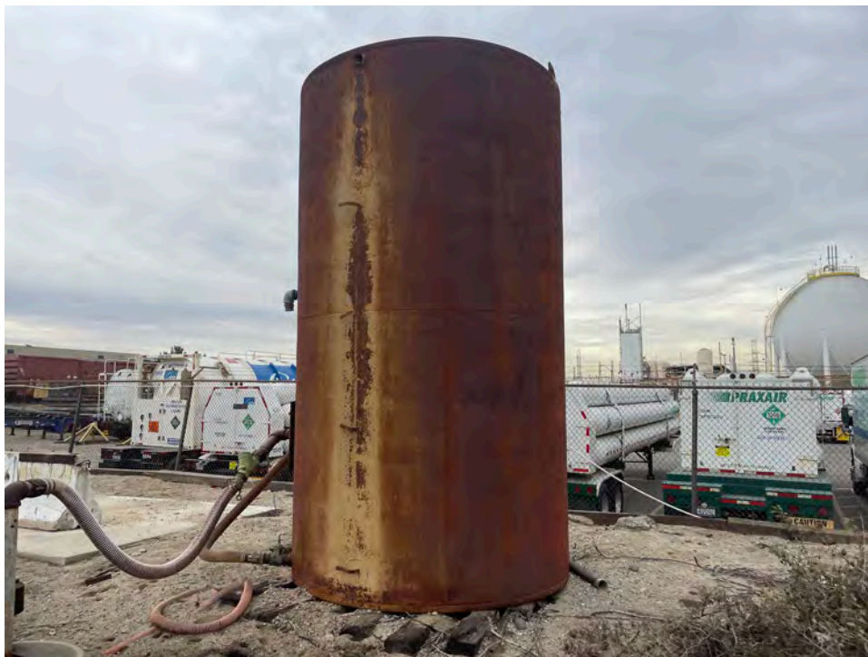
Photograph 2: Wash water storage tank by truck-washing area.
