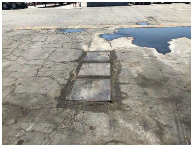
View of three-chamber clarifier in truck washing area.
