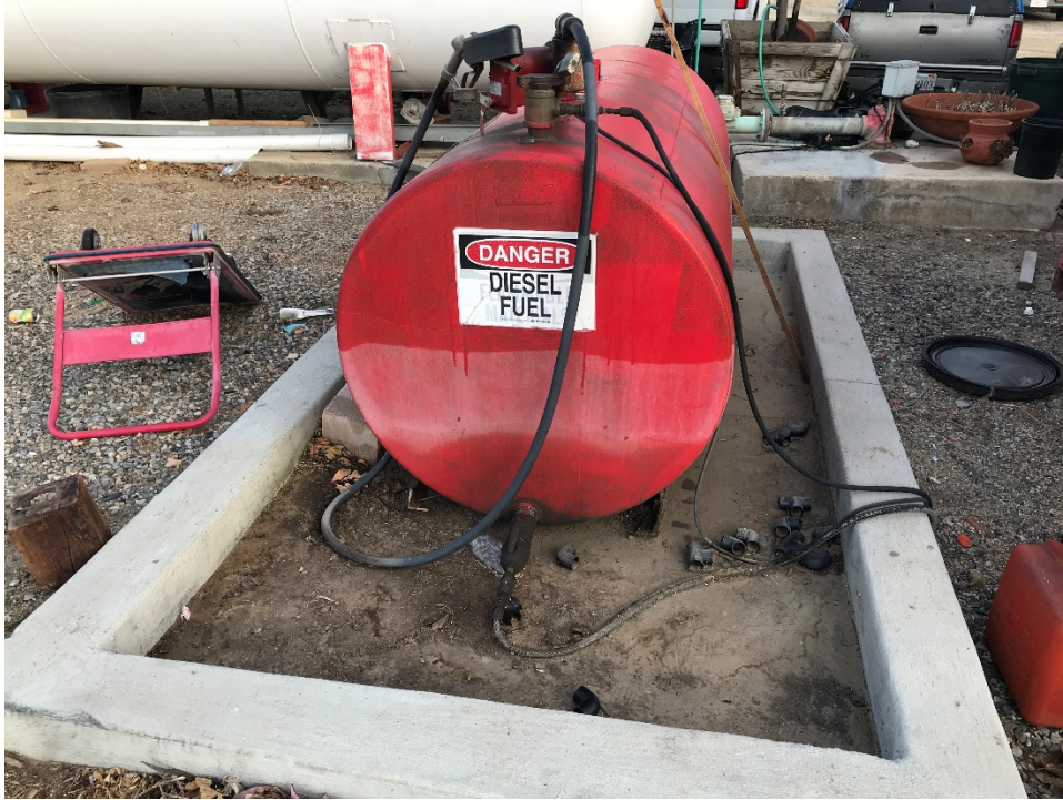
Photo 23 – The diesel fuel AST at the center of the nursery parcel.
