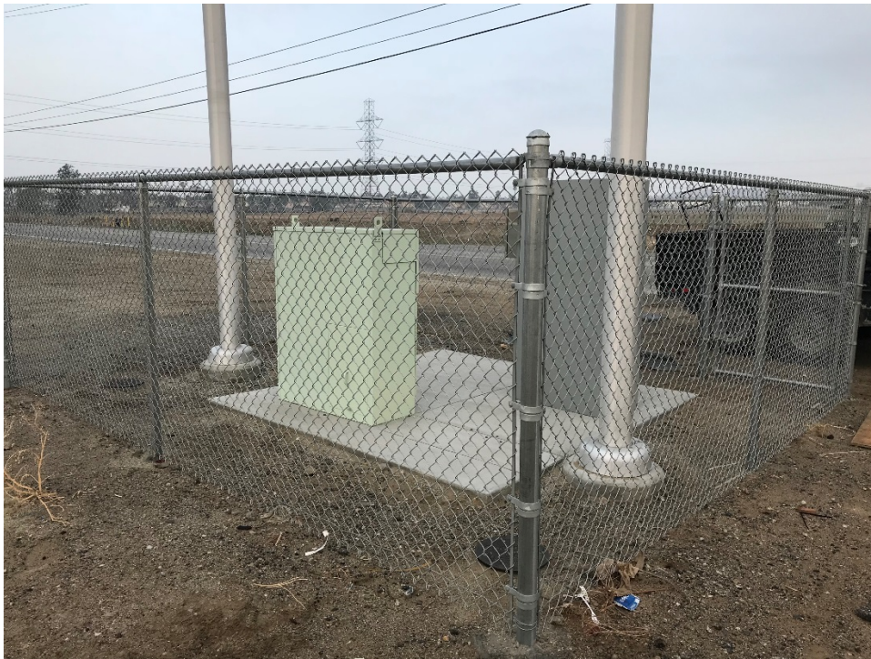
Photo 8 – Remote water monitoring equipment outside the northern end of the Property.
