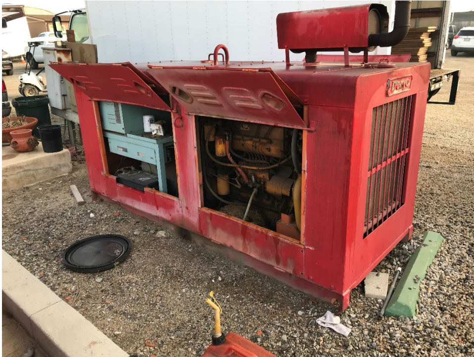
Photo 24 – The emergency generator to the east of the diesel AST.
