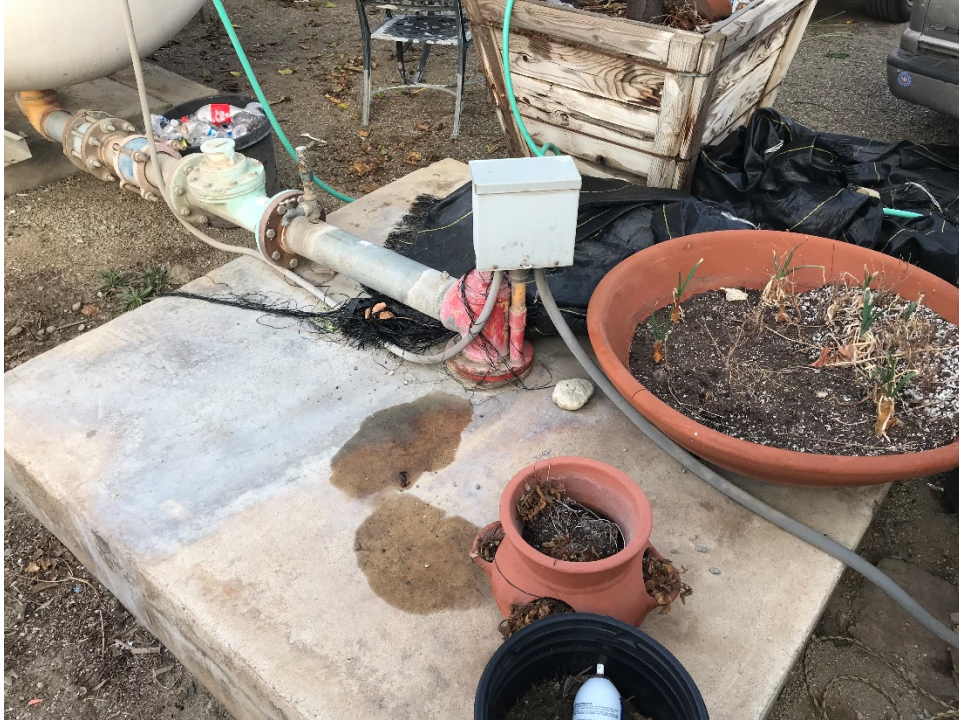
Photo 27 – Groundwater supply well on the center of the Property.
