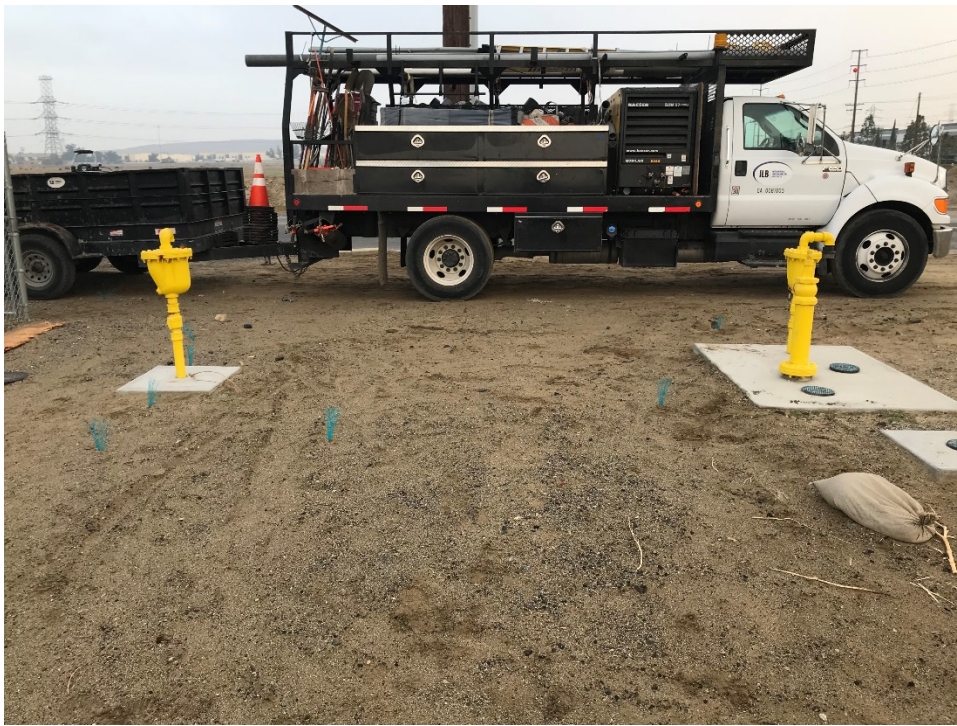
Photo 7 – Water equipment outside the northern edge of the Property.
