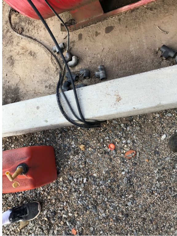
Photo 25 – Area where the fuel line passes outside the berm and underground to the generator.
