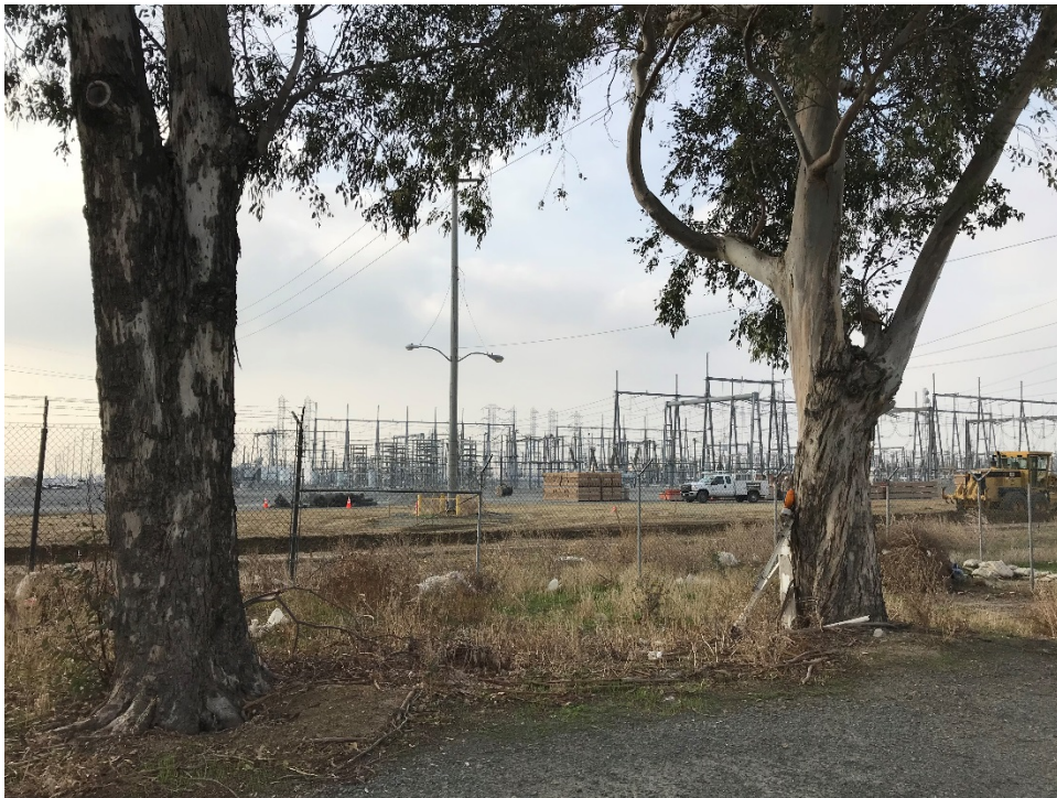
Photo 30 – Electrical substation to the south of the Property.
