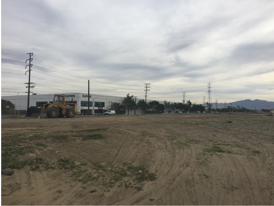
Photo 3 – View showing the eastern side of the northern parcel after the piles were removed on January 30, 2018.
