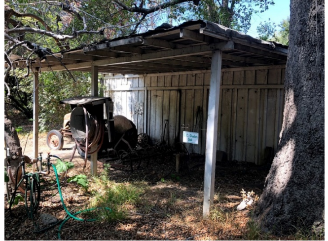
Image 18. View of the south elevation of the Graber Shed building (Resource No. 11).
