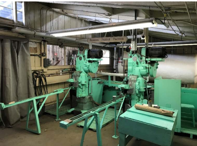
Image 7. The two Panama Paddle Packers machines (Resource No. 22) located on the Canning Room of building resource No.2.
