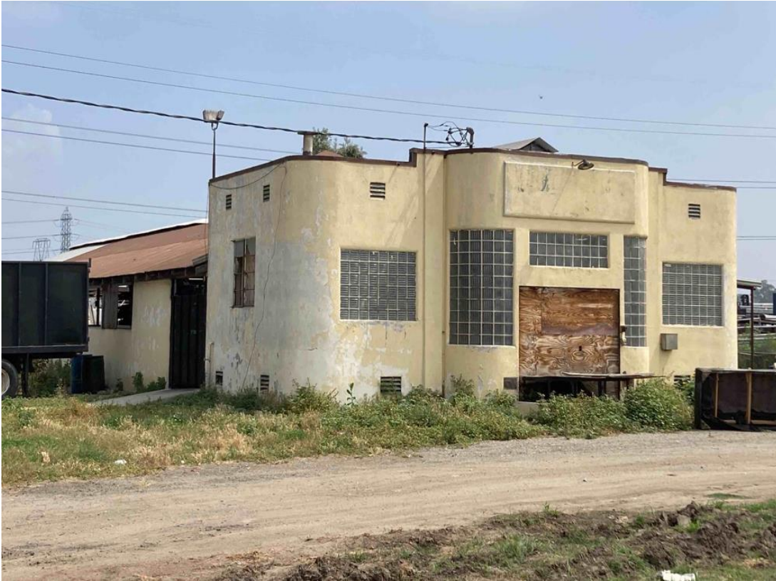
Photograph 4: Edison Avenue milking parlor, west and south elevations, camera facing northeast, May 22, 2023.
