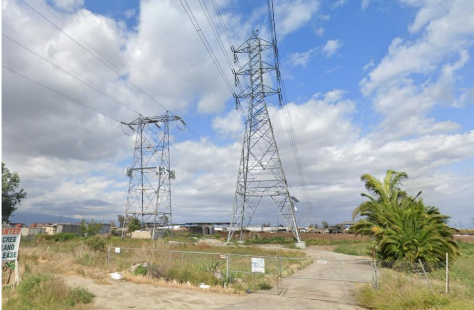
Photo 1: Overview of Transmission Line, View NE.
