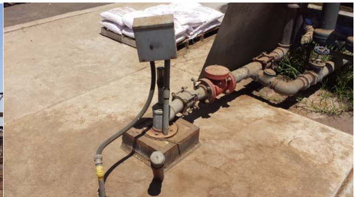
View of well water tank
