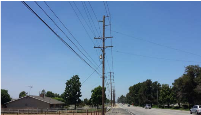
View of pole-mounted transformer on north border of the Property
