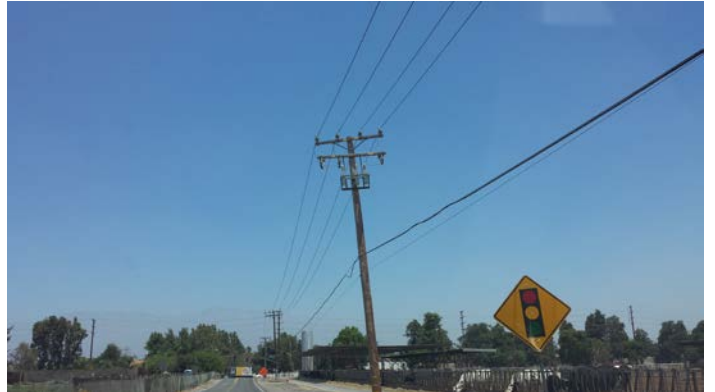
View of pole-mounted transformer on eastern portion of the Property
