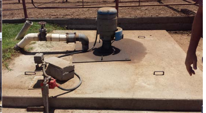
View of reclaimed water underground storage tank
