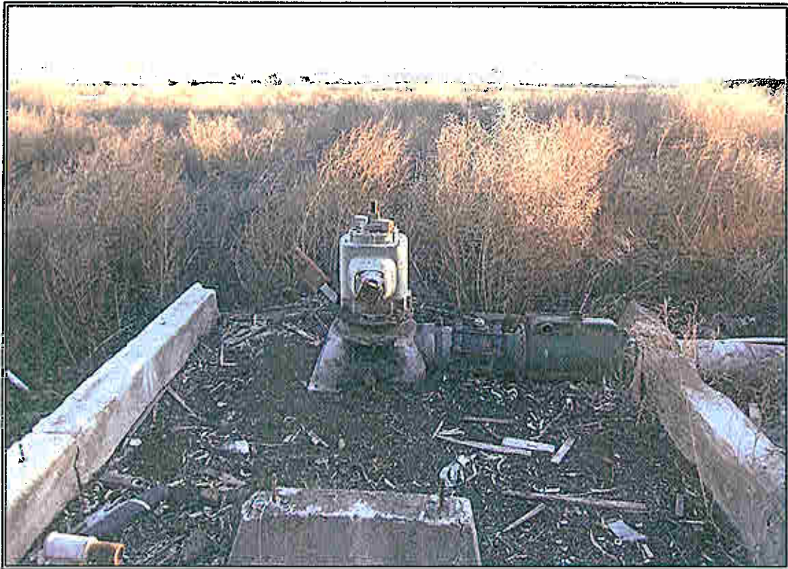
Well on the east side of the site, south of Eucalyptus Avenue.
