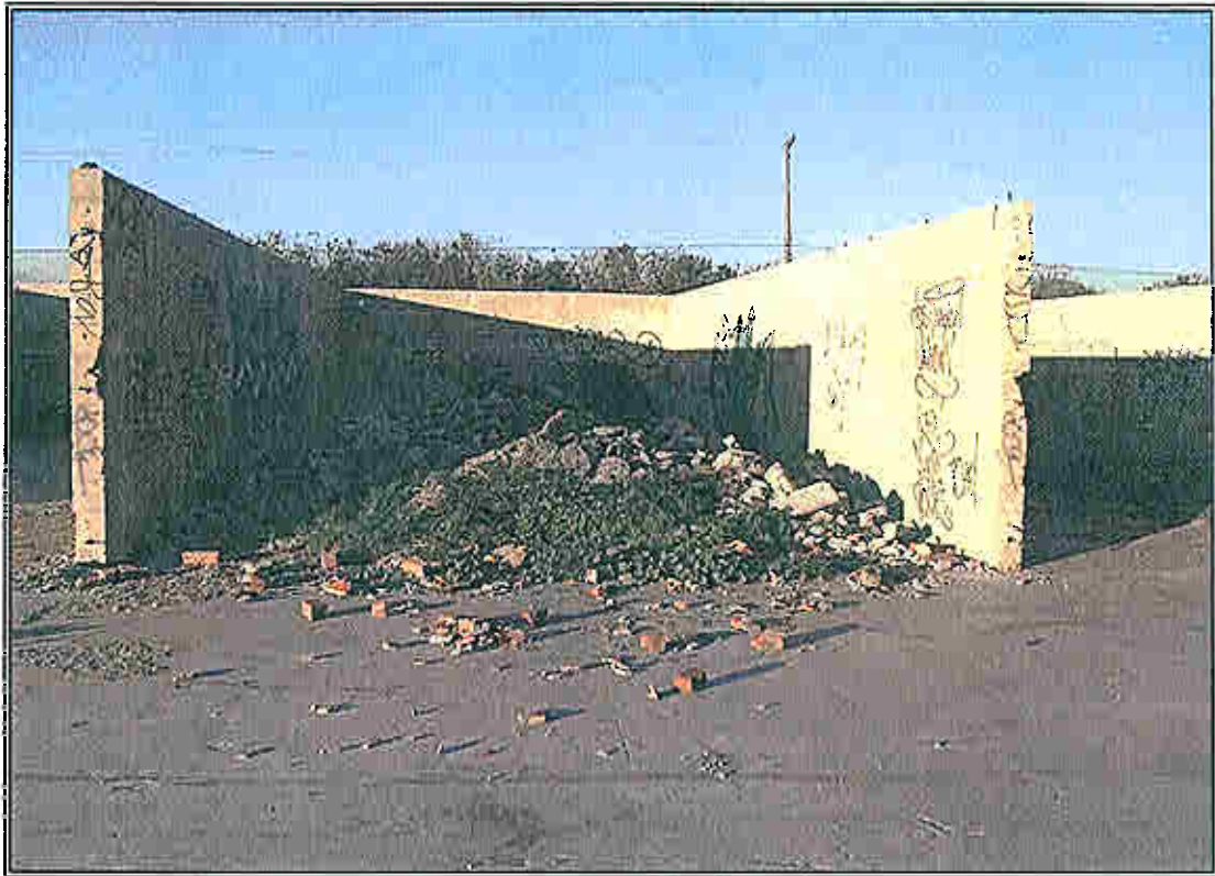
Debris pile of dirt, concrete and asphalt in former grain storage area.
