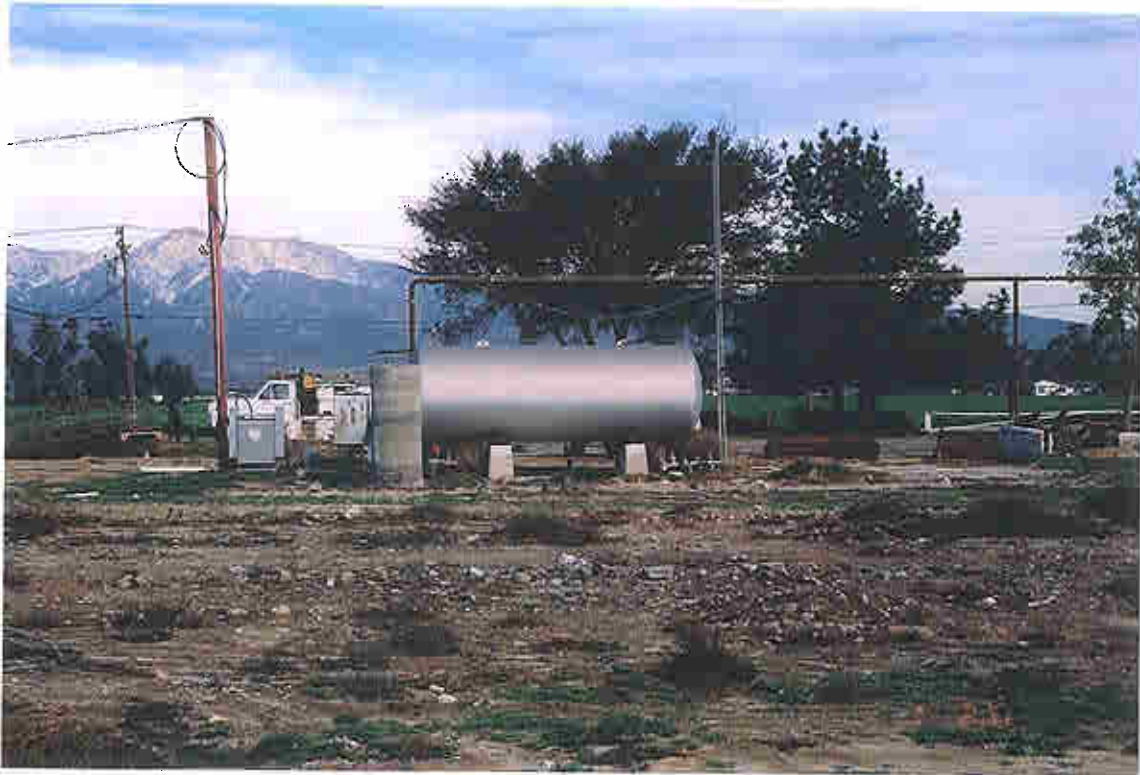
Photo 11 - Water tank, electrical power supply and piping. Located on south side of Eucalyptus Ave.
