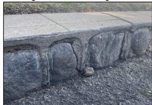
Figure 1: Original Rock Curb
