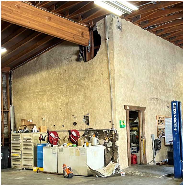
G-11. Wall deterioration observed in the secondary building (8/29/2022).
