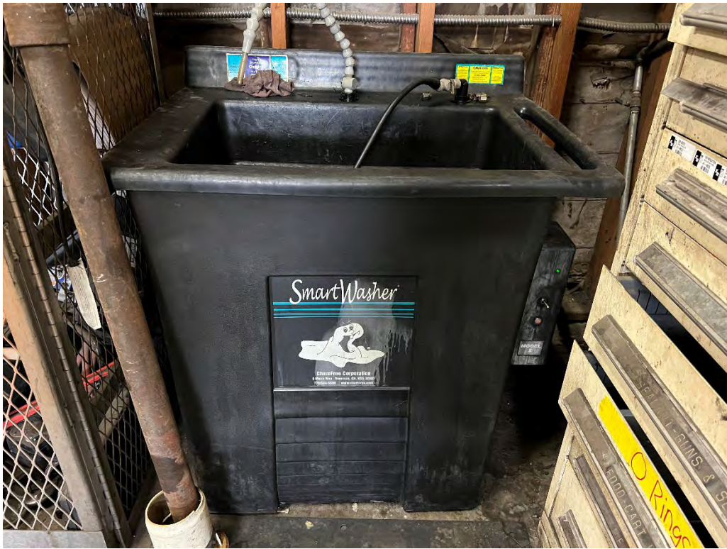
G-9. Vehicle parts washing station observed in secondary building (8/29/2022).
