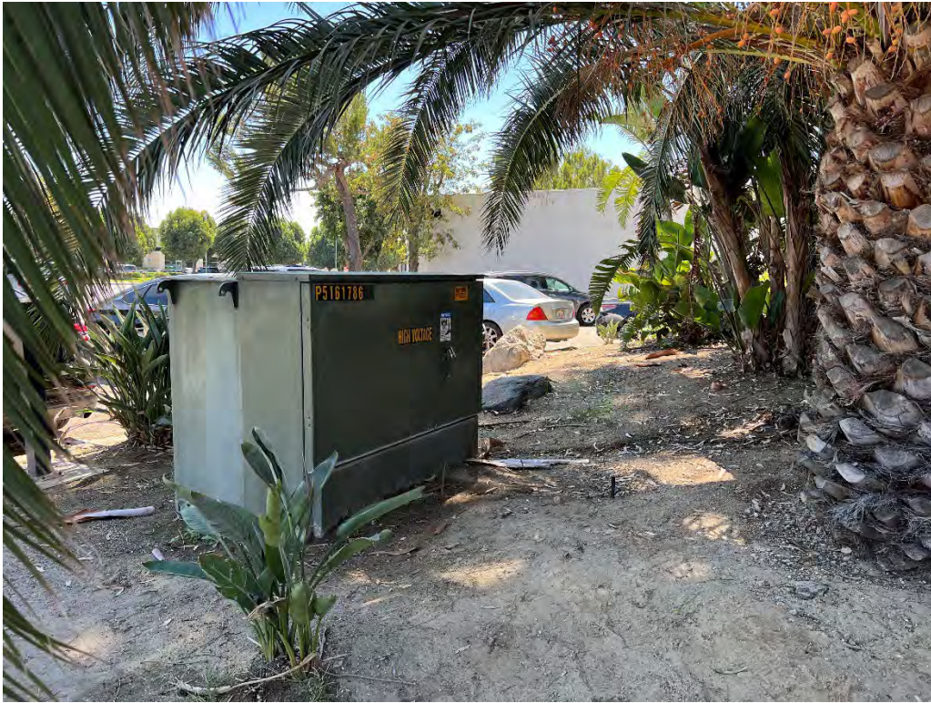
G-1. View of the electrical transformer located in the southeastern portion of the Subject Property (8/29/2022).
