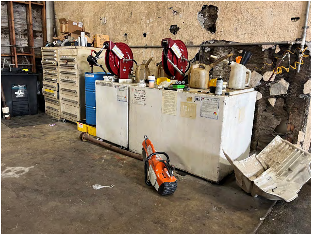
G-8. 240-gallon diesel and 120-gallon motor oil ASTs in secondary building (8/29/2022).
