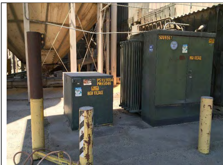
23. View of 1 of 2 SCE Pad-Mounted Transformer labeled with No PCBs
