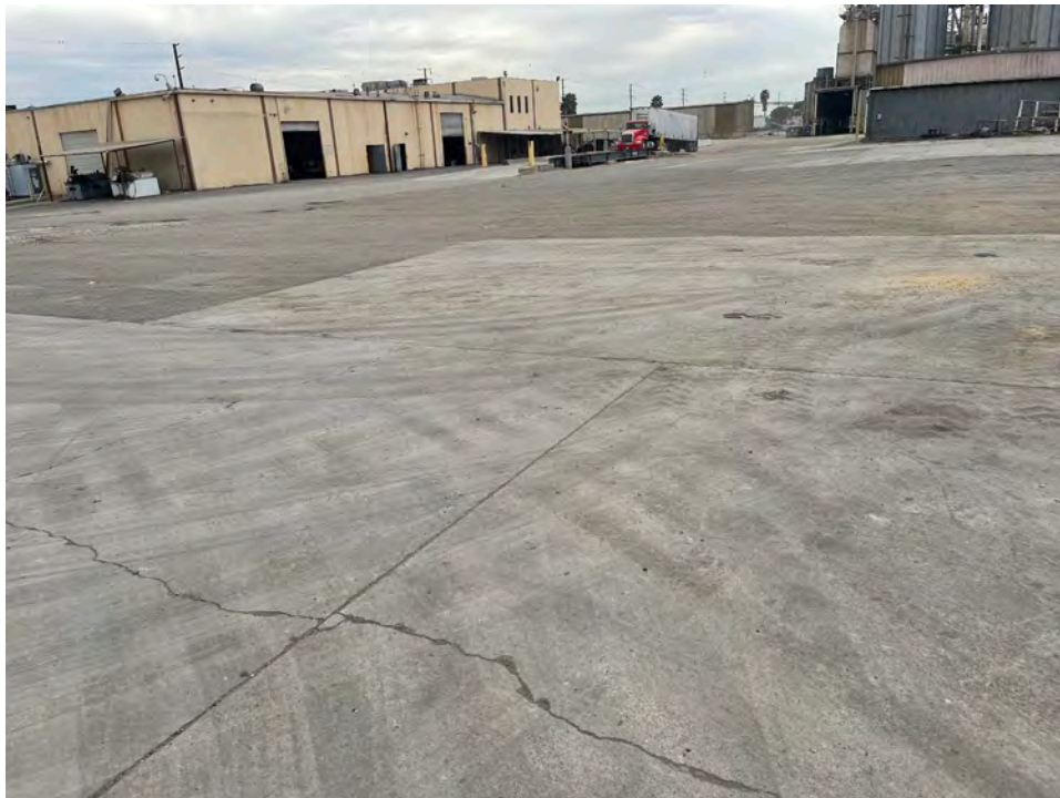
Photograph 6: Former underground storage tank area by Building B.
