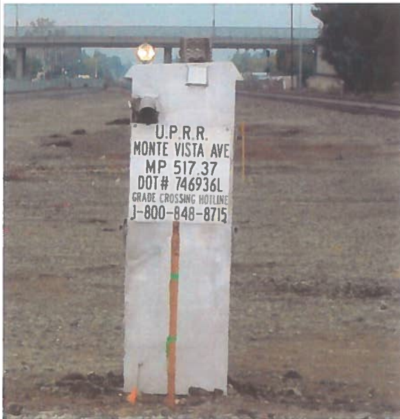
Southern Pacific Railroad at Monte Vista Avenue: signal box. View: W. November, 2012.
