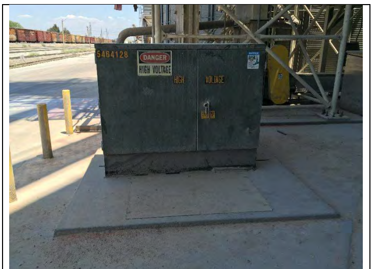
24. View of 2 of 2 SCE Pad-Mounted Transformer labeled with No PCBs
