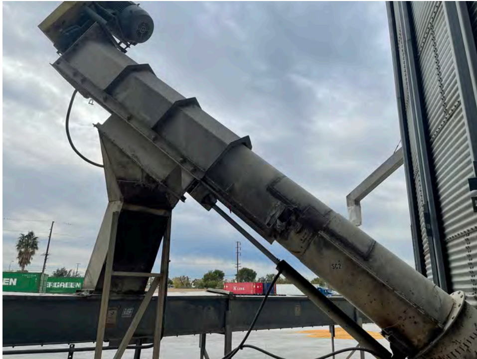
Photograph 9: Hydraulic augers at Scoular grain storage silos.
