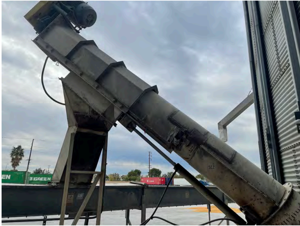
Photograph 9: Hydraulic augers at Scoular grain storage silos.
